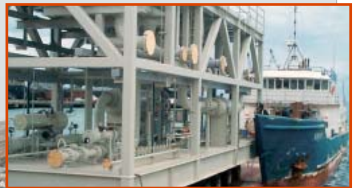
Top: 140T Compressor Skid.
